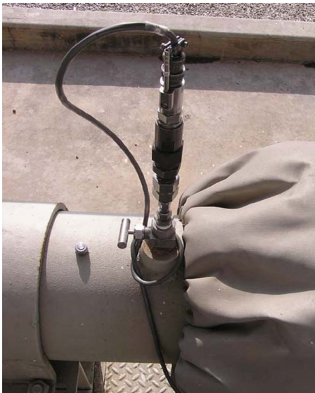
Fig. 5 High frequency pressure transducer in discharge pipe
